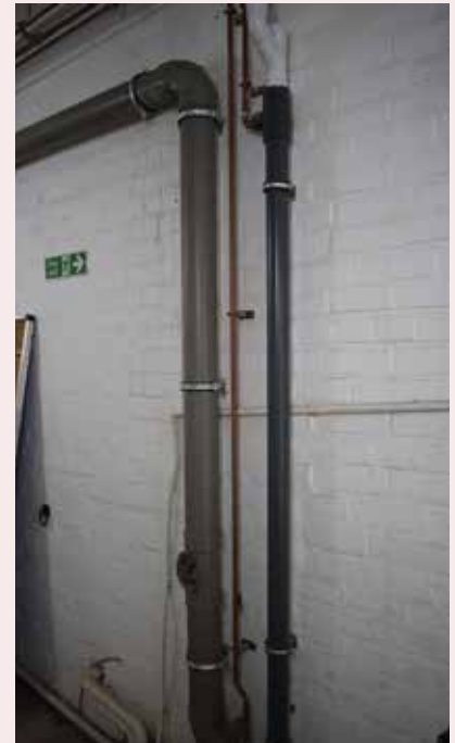
New Water Heat Recovery System leading to the en-suite showers in the Besse Building
